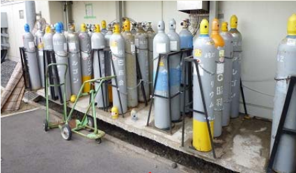
gas cylinder station
