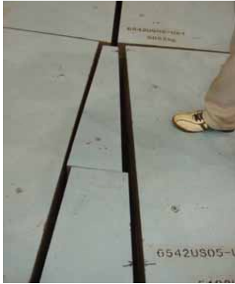
Displacement of shielding walls in MLF 1 st Hall: BL04 Area (left) 2 nd Hall: BL20 Area (right top)
