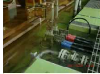
Submerged cables and connectors
