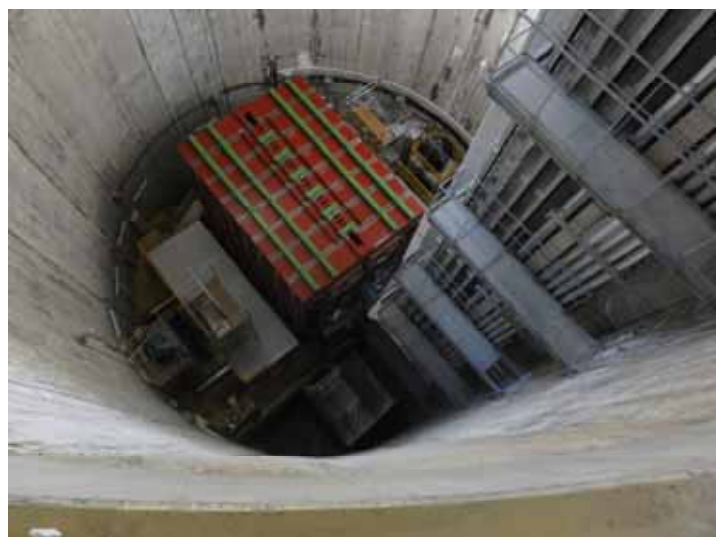
No significant damages through outside inspection. About 1 cm deep water at the bottom. This problem has been already solved.
