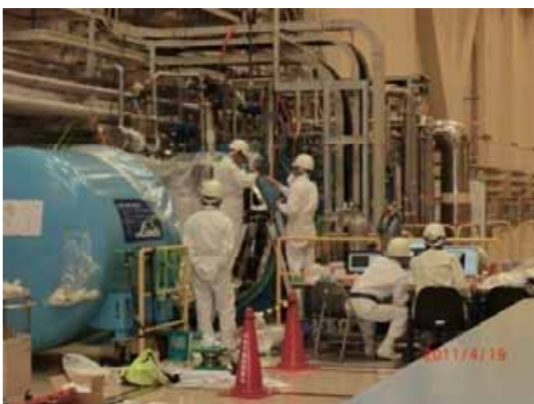
Inspection of Expansion Turbine
